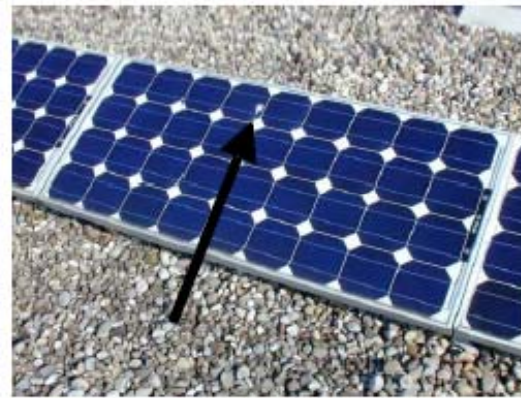
Fig. 13: Bird dropping stays after a heavy rainfall (ewz)
