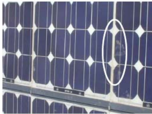
Fig. 12: Some dirt stays after a heavy rainfall (ewz)
